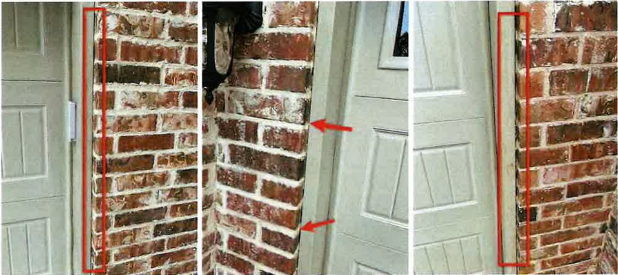
Garage door metal frame has major caulk deterioration around all sides
