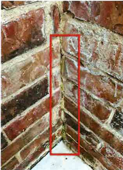
Where retaining wall connects to west corner of home. Moss or microbial growth noticed on caulk as well as moisture at the base of the wall.
