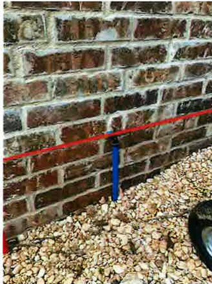
Crack running from front to back on southwest side of home about 20 feet long continuous.
