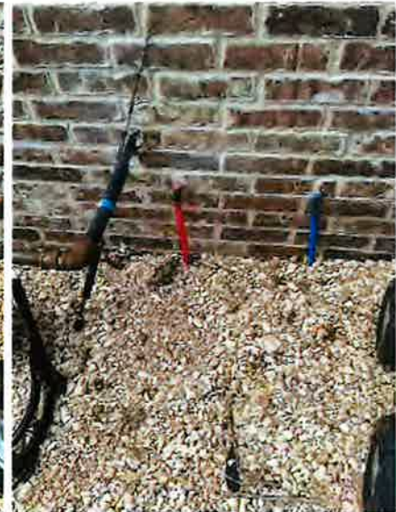
Southwest side of home has drains running right down next to structure.
