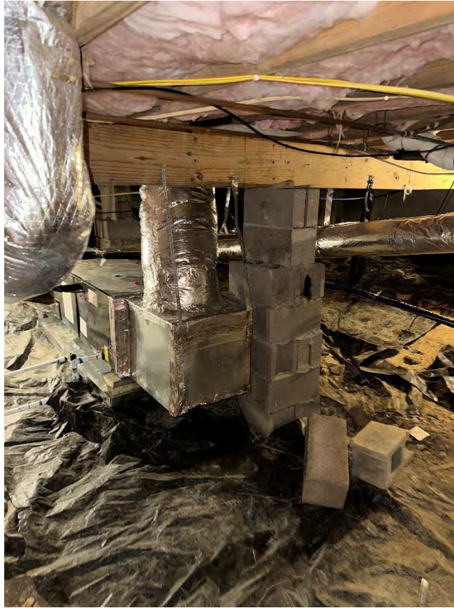
Photo 10. HVAC system and view of current crawlspace vapor barrier
