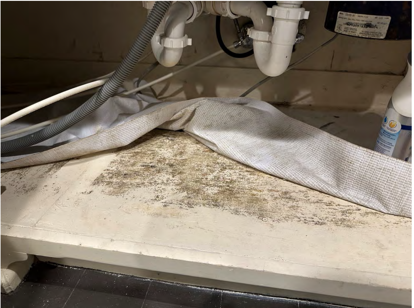
Photo 3. Underneath kitchen cabinetry housing the kitchen sink illustrating visible mold growth
