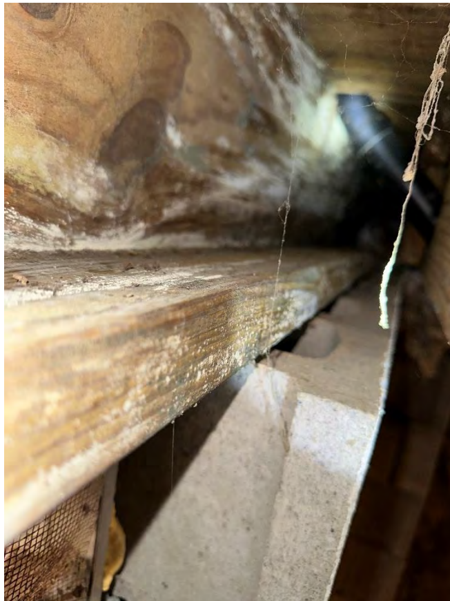
Photo 9. View 2 of crawlspace substructure near kitchen drainage pipe illustrating visible mold growth and moisture staining
