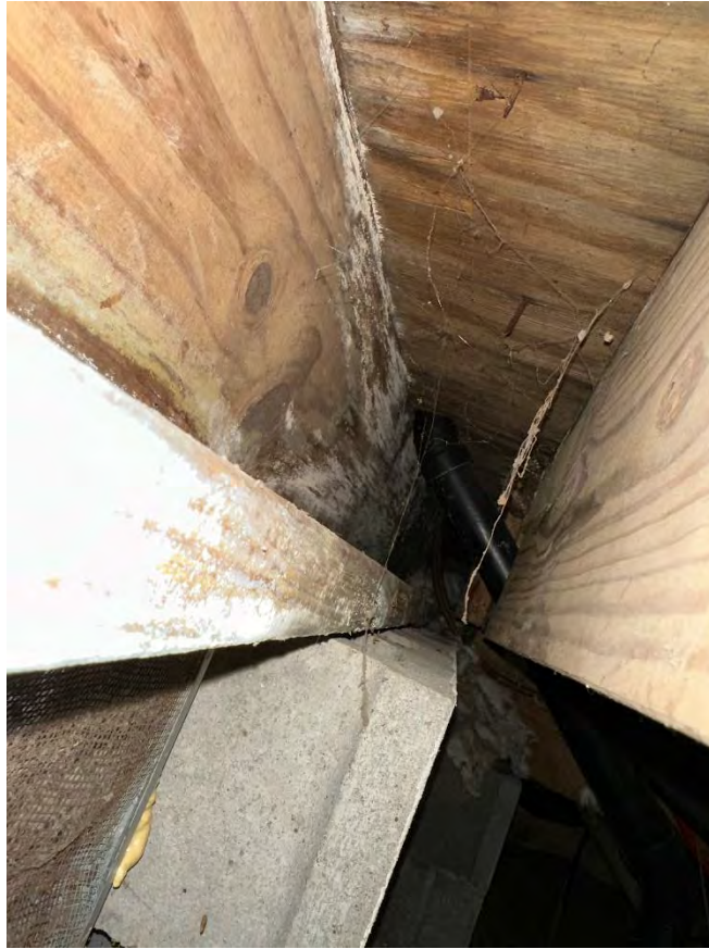
Photo 8. View of crawlspace substructure near kitchen drainage pipe illustrating visible mold growth and moisture staining
