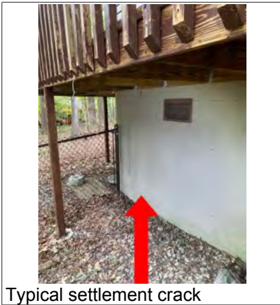
Typical settlement crack
