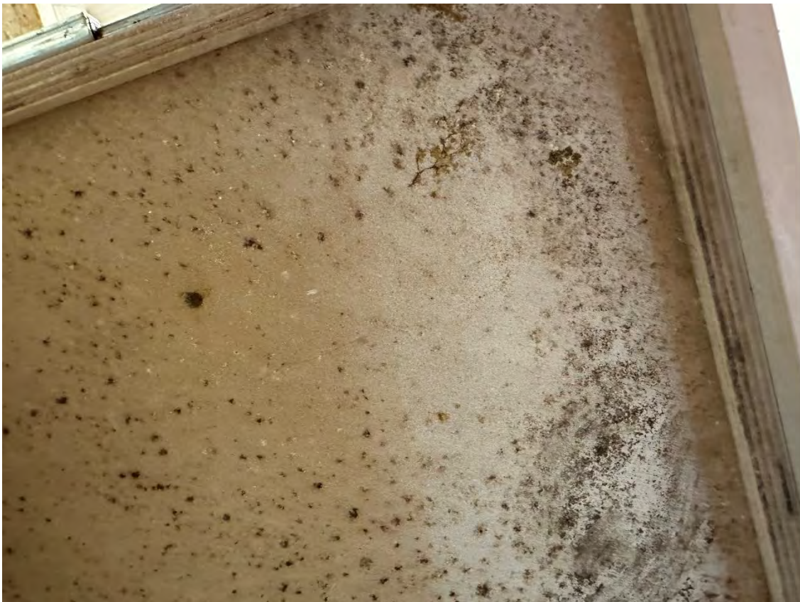
Photo 5. Underside of kitchen cabinet drawer illustrating visible mold growth
